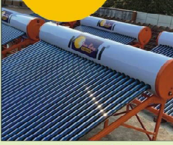
Solar Water Heater Colaco Hospital Mangalore
