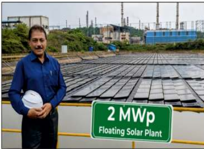
Floating Solar Power Plant
